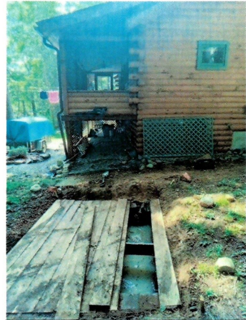
Cesspool for wastewater treatment found in the Town of Hage. Such systems are not allowed by NYS health code
